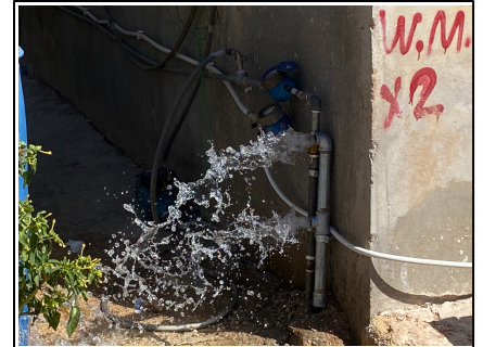
Broken pipe representing physical non-revenue water loss, USAID MESC II
